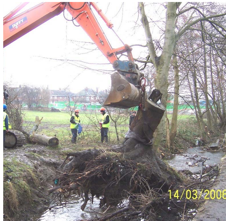
Removal of a mature tree from the centre of Wyke Beck (behind the Foxwoods) as part of the planned maintenance. Flooding in May 2005 affected properties adjacent to this stretch of beck
