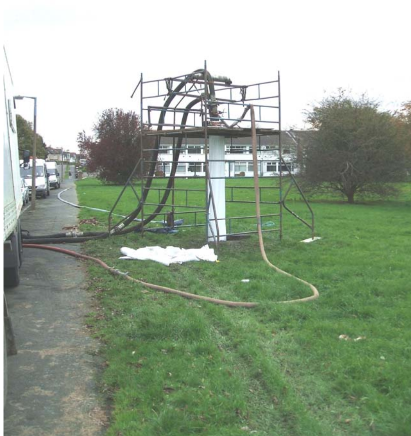
Rig set up for hot cured resin lining of culvert at High Moor Avenue (Moortown)
